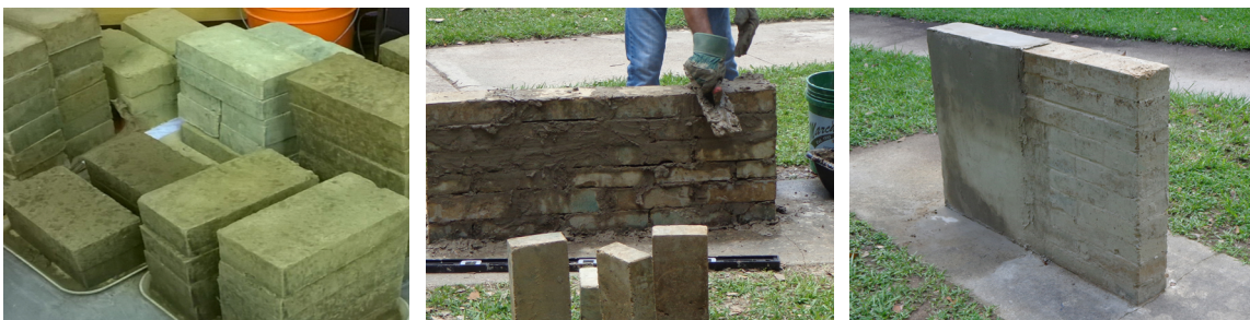
Figure 4: Earth block wall components and construction: earth blocks (left), wall during construction (center), and completed wall (right). Source: (Author)
