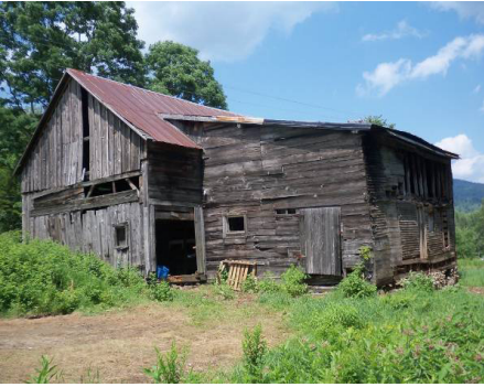
Photo 2: View of barn from the Southeast with secondary structure to be removed on the right
